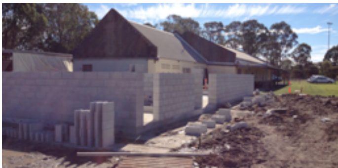
2013: Blockwork in progress on the new dressing rooms at Willawong in June, and, right, children taking part in Go Games in July.
